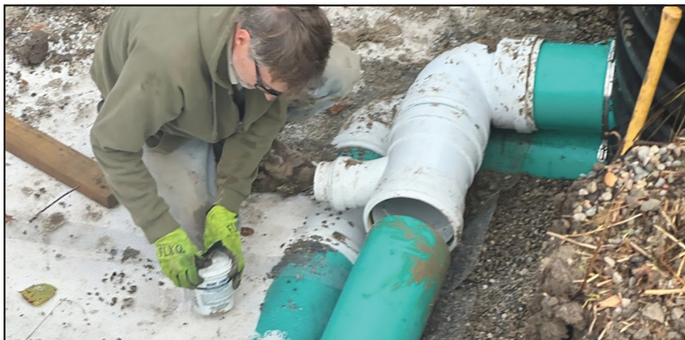
A worker helps install a phosphorus filter in northwest Ohio's Defiance County. A small fraction of farm fields in the region are disproportionately responsible for a lot of phosphorus pollution.
